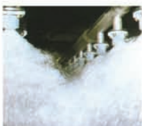
Tower desulfurization in power station
